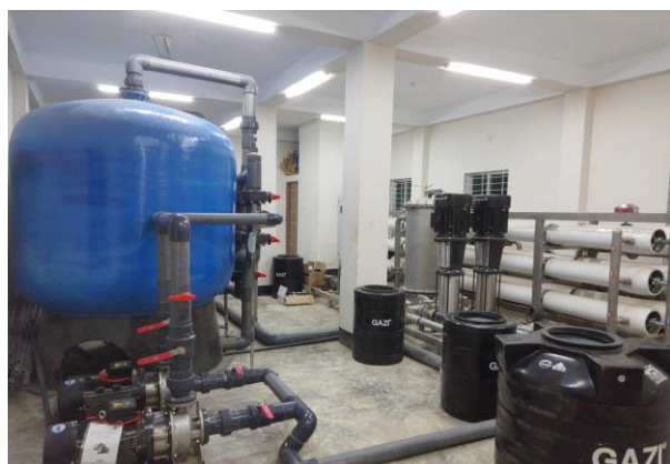
Recently built water treatment plant (supported by IDCB Project, Phase-II) which will be enabled to supply fresh water in the residential area
