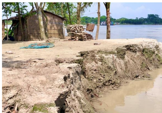
A view of River Bank failure in the project area
